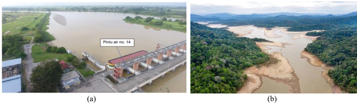
Figure 2. (a) Failure of Gate 14 at the Sungai Muda Barrage, (b) Low water level at Sungai Muda on 14 May 2023
